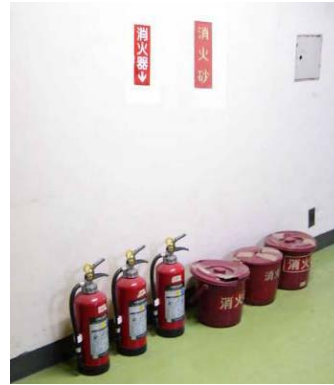
Fire extinguishers are located in corridors (Some are located in rooms)
