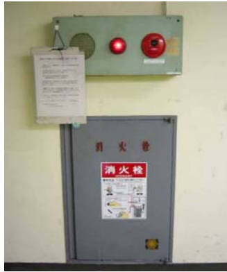
Fire alarm (top) and fire hydrant (below)
