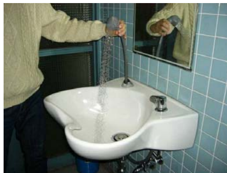
Emergency showers (located in washrooms)
